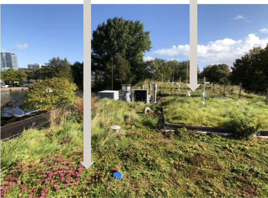
Conventional green roof
